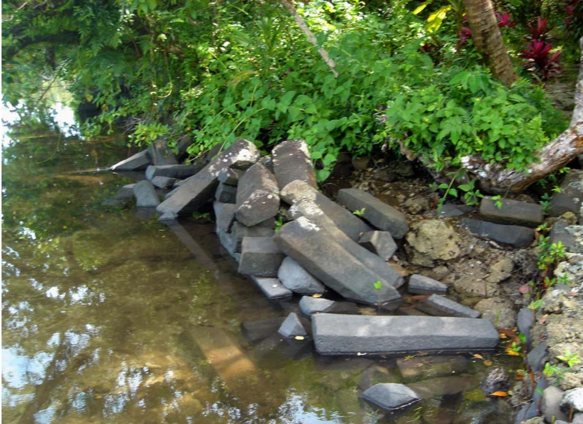
Figure III-1. View of exterior of one of the Nan Madol artificial islets, Usendau (UED), showing displacement of columnar header and stretcher construction and exposed coral rubble fill behind this retaining wall. This kind of deterioration and damage weakens the wall itself and results in deflation of the islet fill from tidal action. [photo nm_ued_shoreline_00334; k. seikel]
